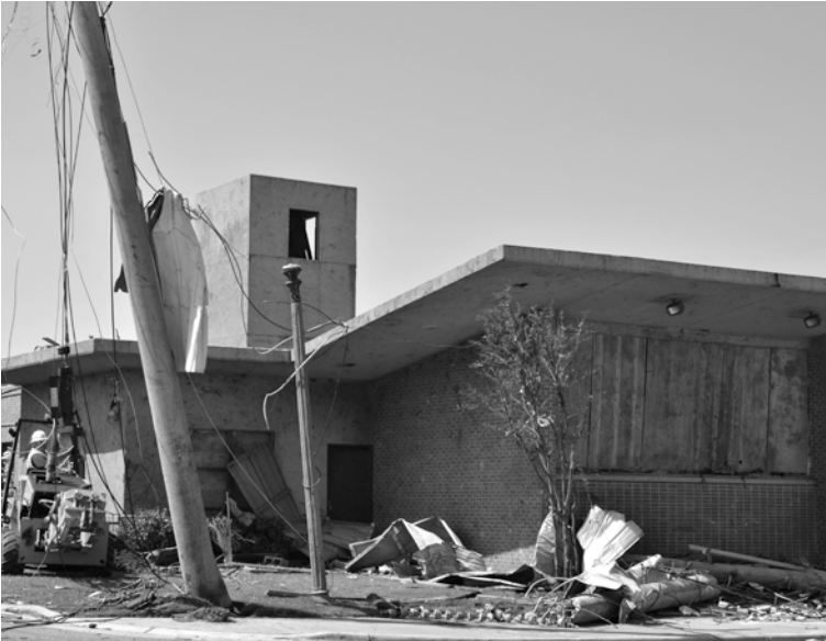
Tuscaloosa's Fire Station 4 was heavily damaged by the April 27th tornado.
